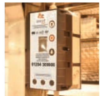
direct drive control panel
