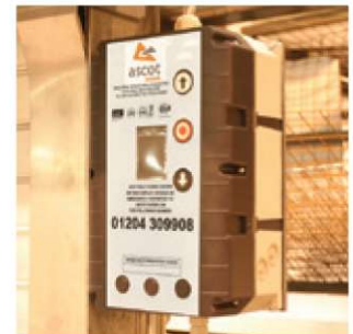
direct drive control panel
